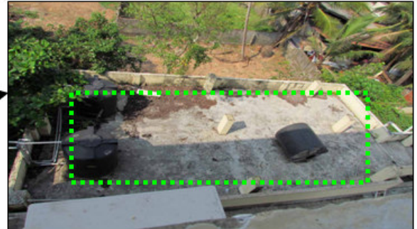
Aerial view of the construction site ( Approx area 750 sq feet (Dimensions 12 m x 6 m)
